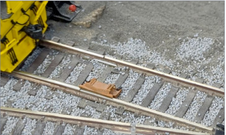
6. Derail in closed position.
