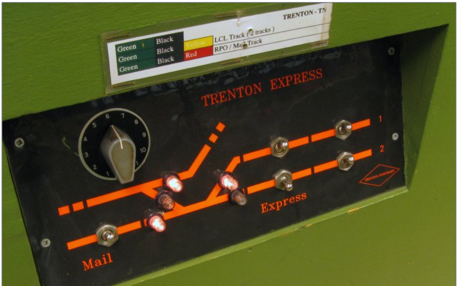
4. The Trenton express control panel.
