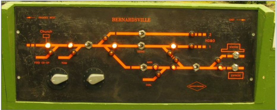
2. Bernardsville control panel (TN).
