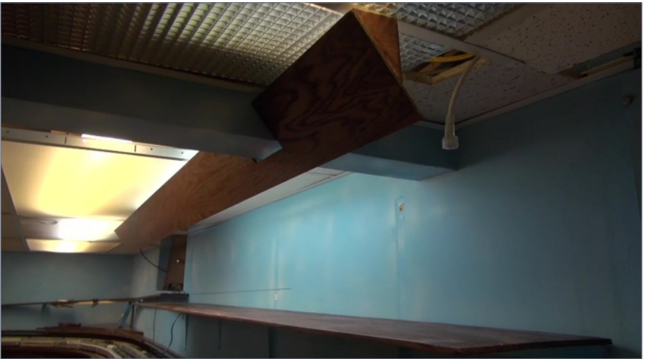
6. To add light to the shelf the module is on, Ken installs an angled valence. He'll install an LED light string later.
