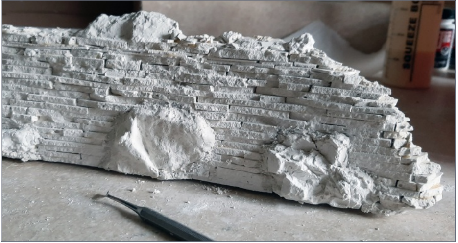
12. Rock castings made from commercial molds are glued onto the wall and the seams patched with plaster.
