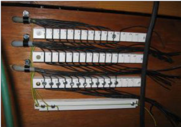
17. Main wiring board with three bus cables.
