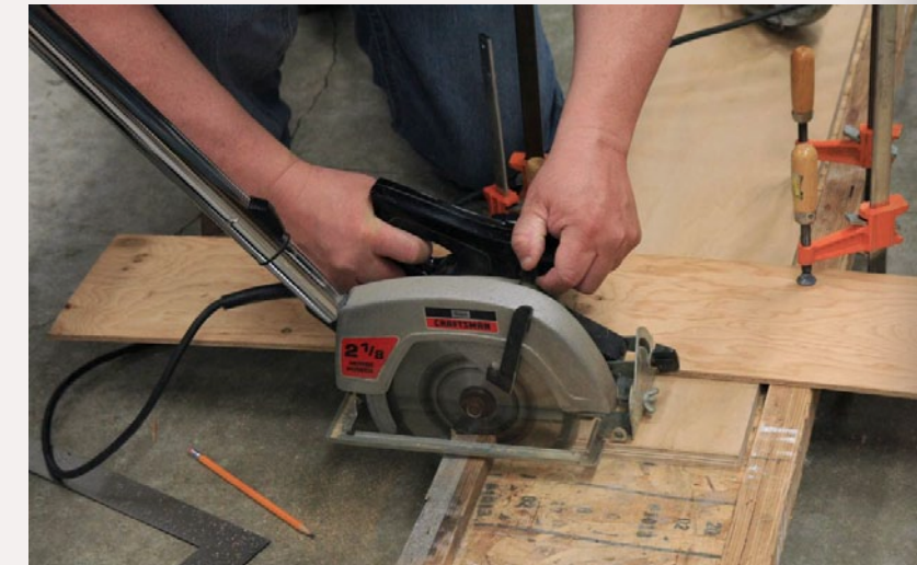
FIGURE 14: cutting the engineered beams to length. Using the vacuum keeps dust generation to a minimum in the train room.
