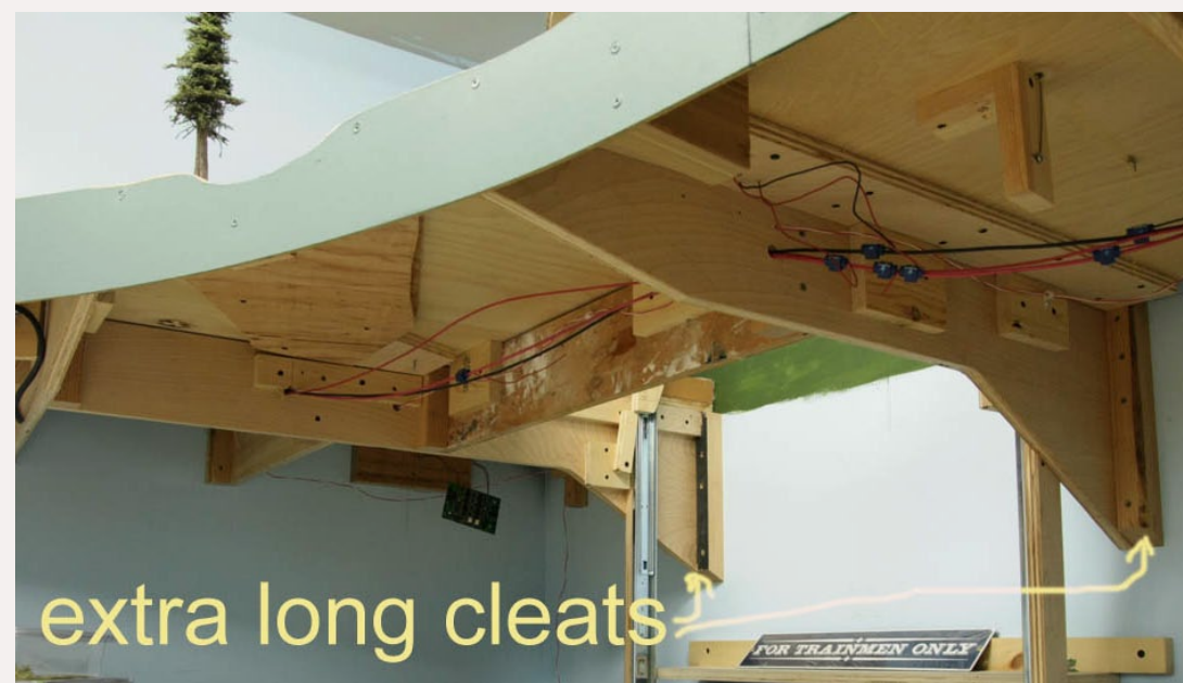
FIGURE 7: Long joists below Oakhill with extra long cleats extending downward.
